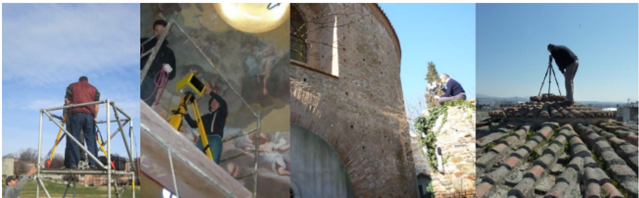
Figure 5-8. 3D Digitisation in progress using a terrestrial 3D range Scanner – Examples of using of temporary scaffolding (Image courtesy [53]-[56])
